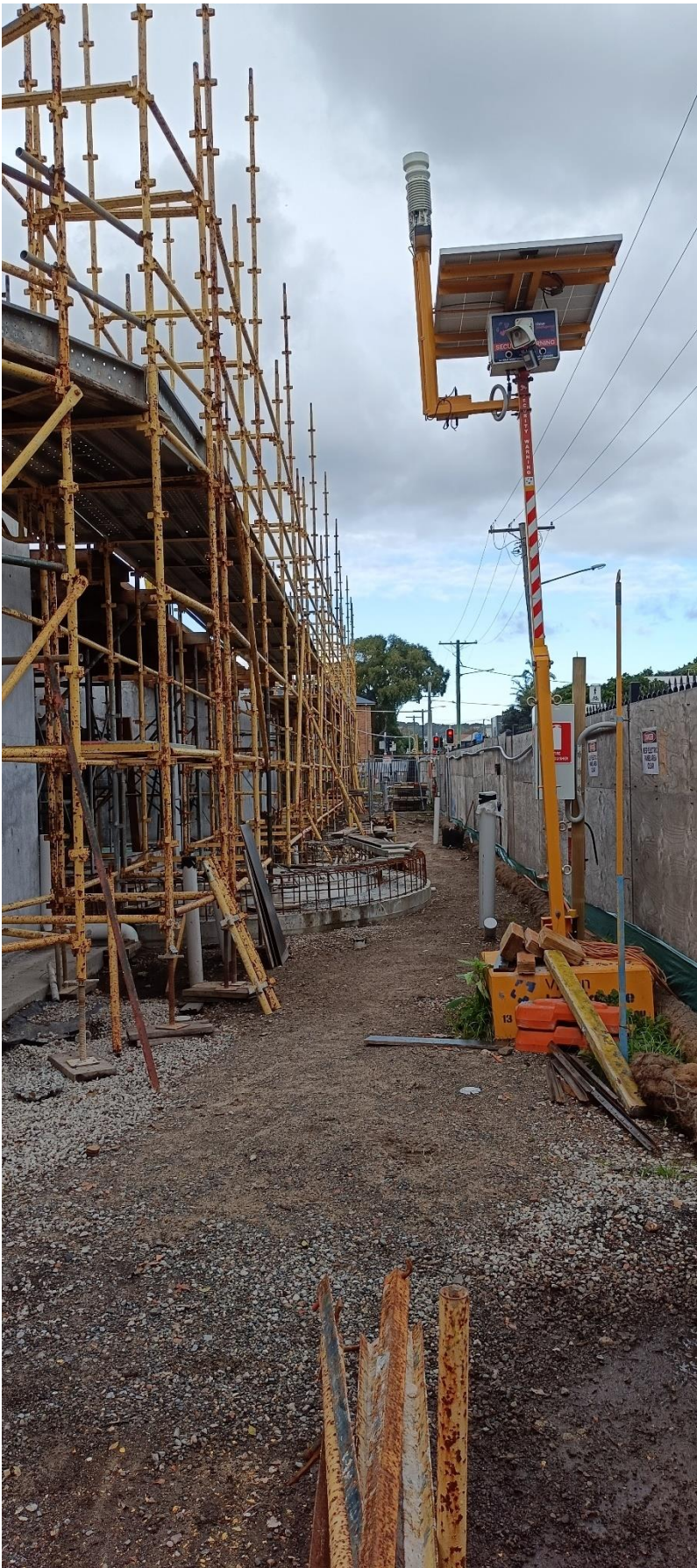
Photograph C.9 Real time noise and weather monitoring in place along Union Street. Erosion controls in place in accordance with ESCP.
